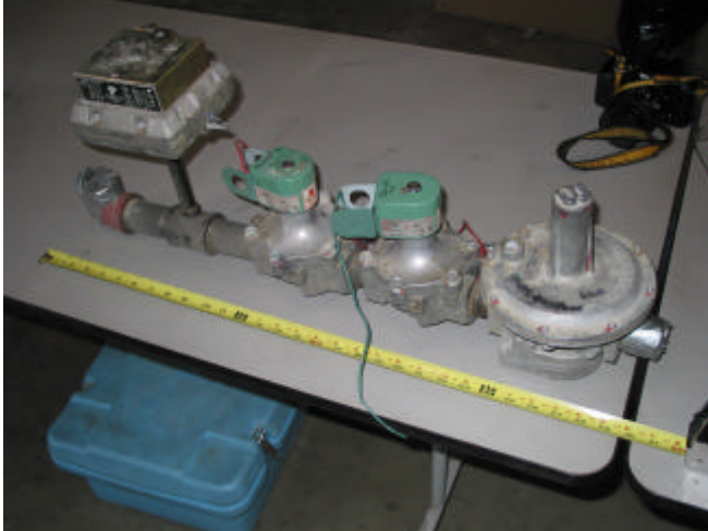
Burner Gas-Control Valve Train
